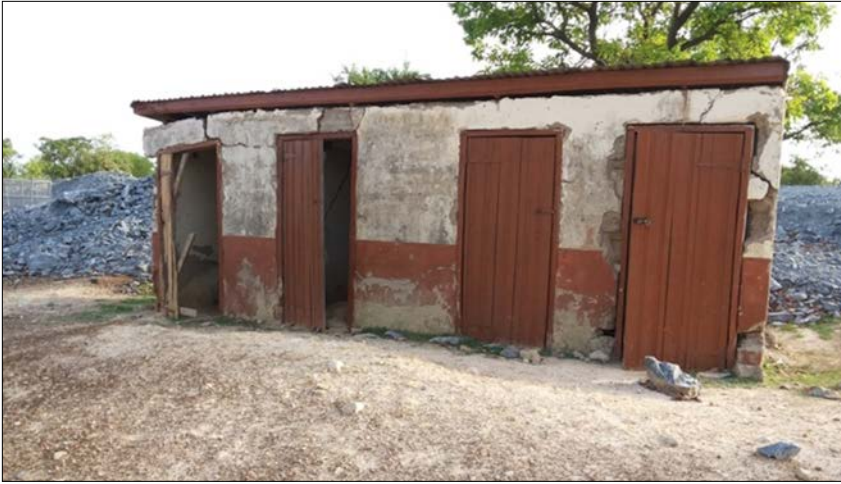
Blasting from Shaanxi damages school's washrooms
