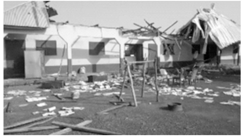
The rainstorm destroyed several buildings
